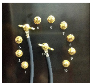
GPS360 Relay Connected to Rectifier AC
