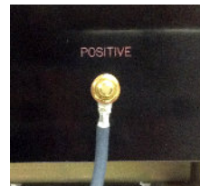
GPS360 Relay Connected to Rectifier Positive
